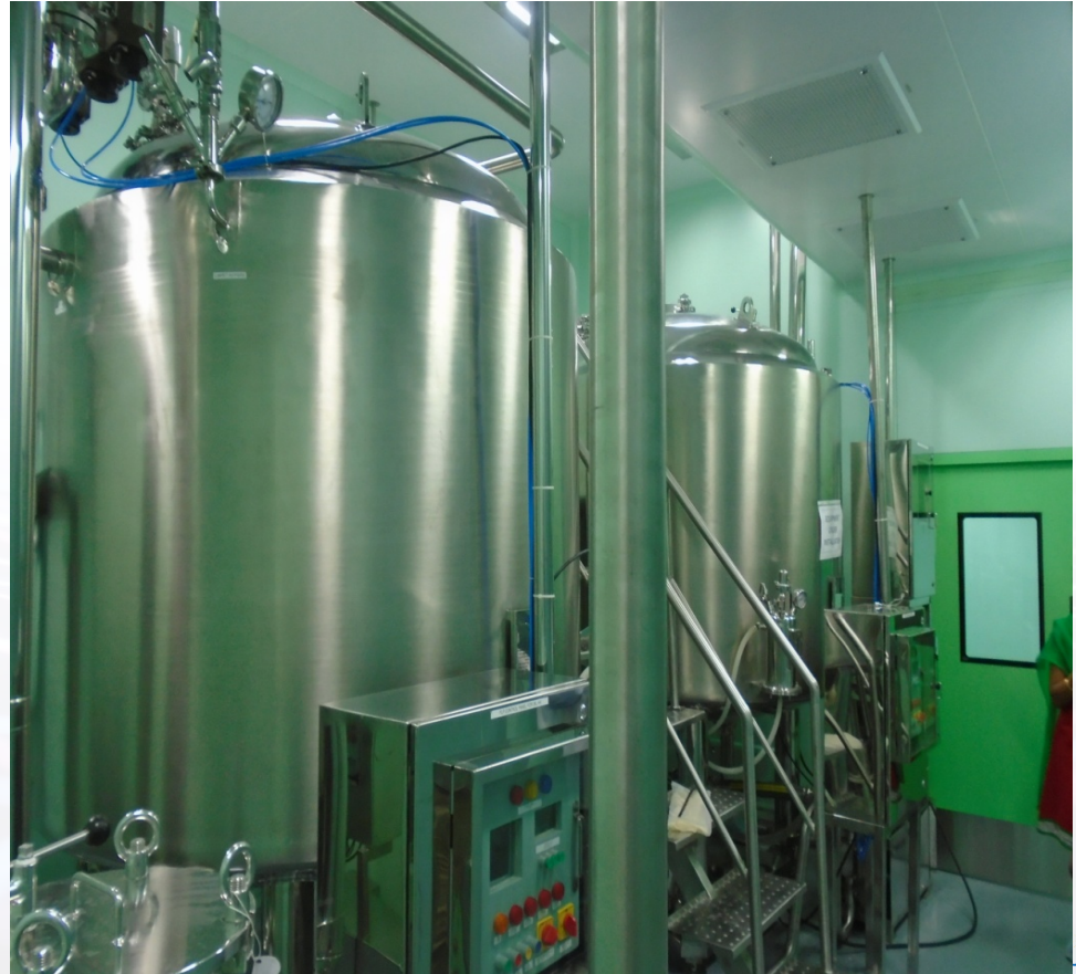
2000L Mixing Tank and 2000L Holding Tank
